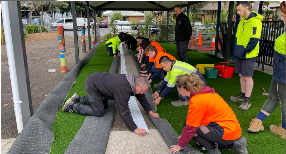
Under the supervision of teachers, David and Zoran , Certificate 1. Agri Food students are learning to lay artificial turf under the new gazebo area.
